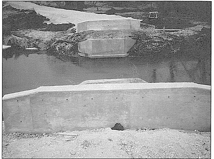
New abutments are ready for installation of bridge across West Branch of DuPage River in Winfield Mounds Forest Preserve. New IPP section heads south to old Chicago, Aurora and Elgin Geneva Spur right-of-way.
