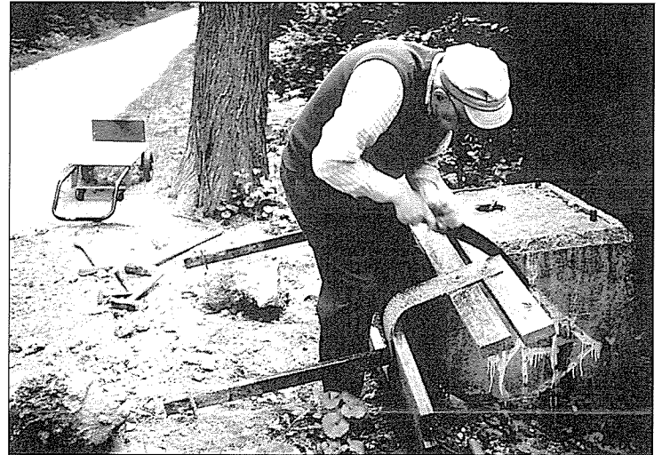
Paul Mooring dismantles vandalized bench near Lake Arrowhead. Large concrete block (right) will have to substitute for bench.
