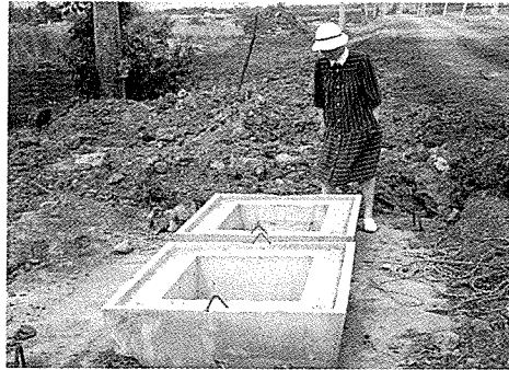
Com Ed owns most of IPP Geneva Spur and has just buried its 34 KV lines at DuPage County Airport. All vegetation has been removed.
