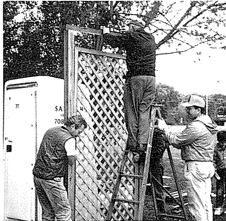
Mark Newell, Paul Mooring and Ken Moss help install decorative wood screen to hide Sani-john on IPP near Warrenville City Hall.
