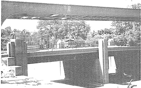
New IPP bridge at Rte. 83 towers over quaint old one, soon to be demolished.
