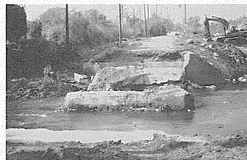
Bridge out at Salt Creek in Elmhurst. IDOT plans to replace before end of year.
