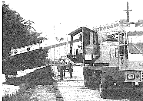
DuPage County DOT crew widens Path between Montclair and Park, Glen Ellyn.
