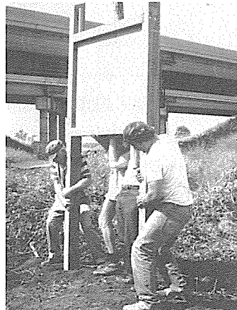
IPP members wrestle sign into place at east end of Batavia Spur bypass. (East-West Tollway bridge in background).
