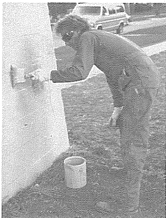
Joe Bremer, Wheaton Public Works Department, paints pier of Volunteer Bridge. The job required more than 15 gallons of paint.
