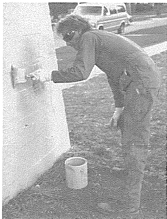
Joe Bremer, Wheaton Public Works Department, paints pier of Volunteer Bridge. The job required more than 15 gallons of paint.
