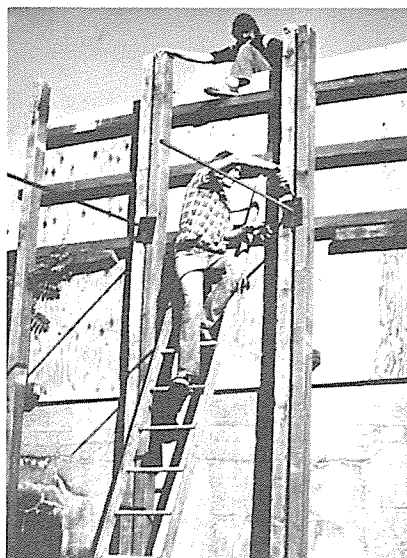
Husband and wife engineering team, Jim and Carol Schumann, remove bolts from concrete forms.
