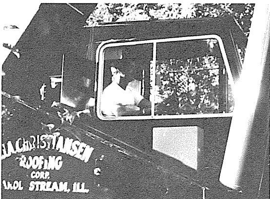
Crane operator Ron Woodward with crane donated by F.J.A. Christiansen Roofing Corp., Carol Stream, pours concrete.
