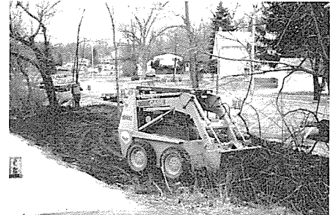
Wheaton Public Works Department crew begins clearing and grading east of President St.
