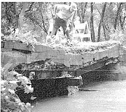
After the flood, Kline Creek bridge, August 16, 1987.
