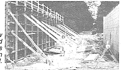
Concrete forms for new Butterfield Road underpass. St. James Farm gate is in background.
