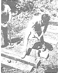
Path members drive re-bar stakes to anchor R.R. tie steps at Blackwell Forest Preserve.
